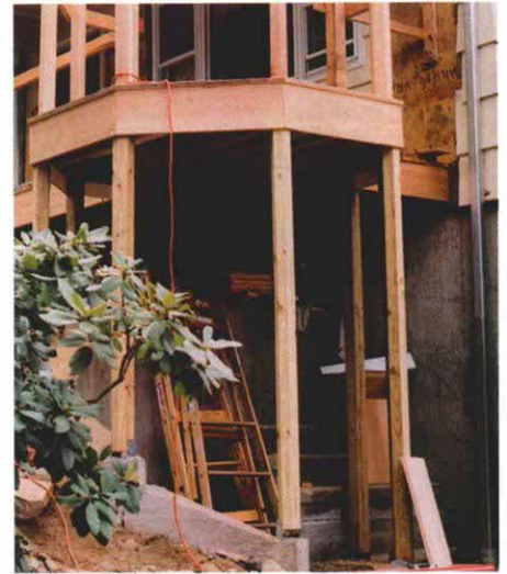
Beveled supports. Posts were milled to continue the octagon down to the retaining wall.
