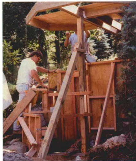
Plumbing the forms. Plumb lines at the deck corners help locate the foundation forms.
